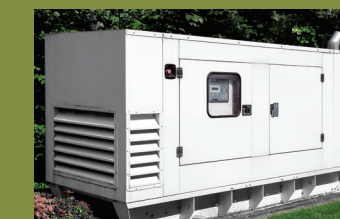
24x7 Power Backup
